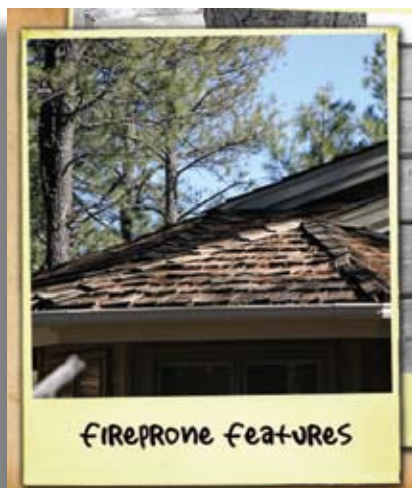
Use of flammable roofing materials
