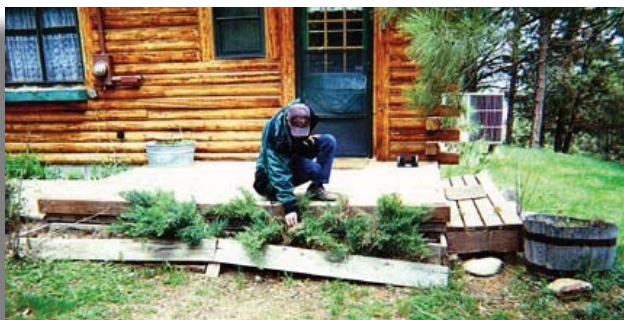
Flammable vegetation in direct contact with house
